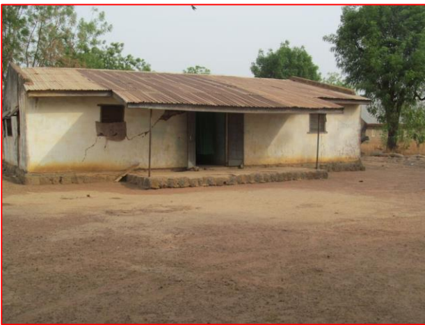
Below: PHC Nagane, in need of major renovation
