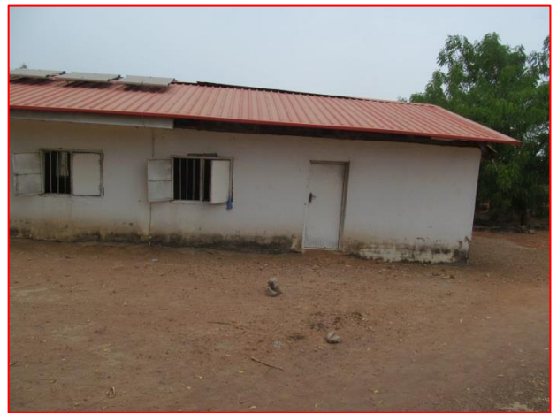
Below: PHC Talgwang, in need of minor renovation
