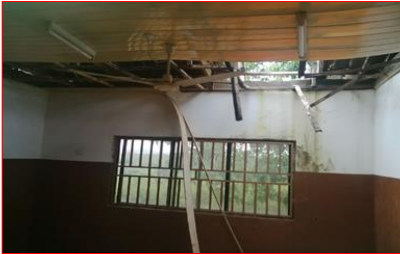
Below: The infrastructural state of HC, Igu, Bwari
