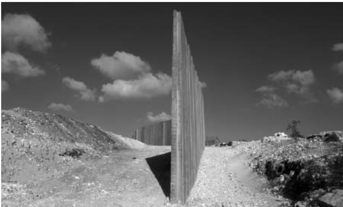
View of the separation barrier under construction near Bethlehem. When it is completed, the movement of Bethlehem residents will be severely restricted
